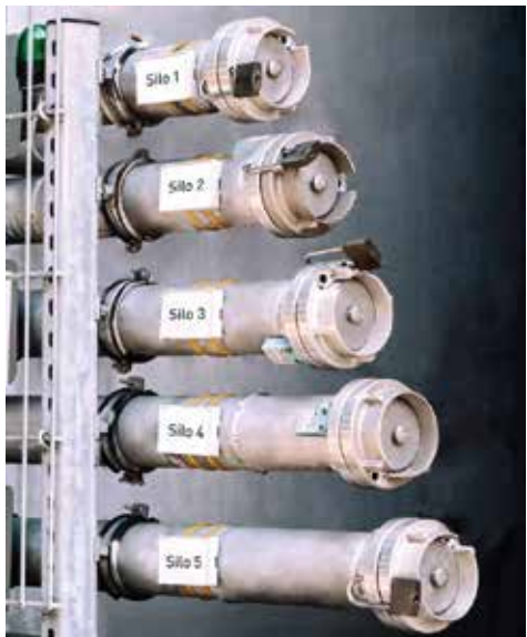
Silo Loading and Transfer lines
